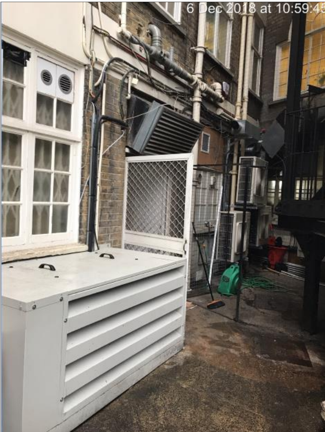
Cold room condenser – photograph taken 6 December 2018
